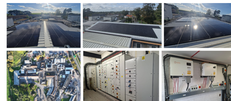
Solar PV Project
